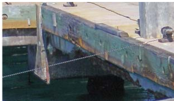
Sections of Kewalo Basin are in need of repair and renovation.
